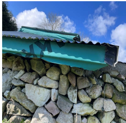
Plate 3-21 Gaps under corrugated roof
