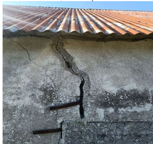
Plate 3-12 Large crack in stonework on northern wall
